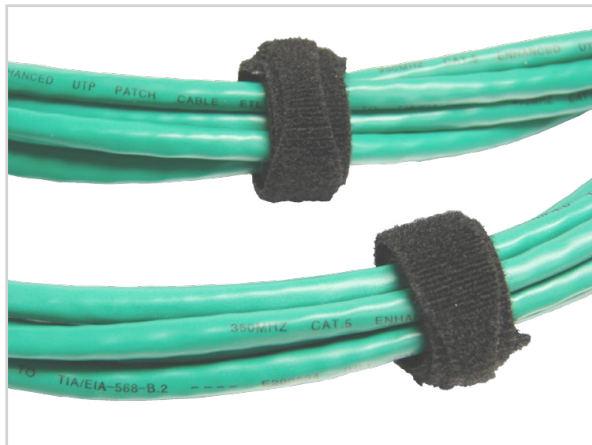
CABLE BUNDLE WITH VELCRO TIES
